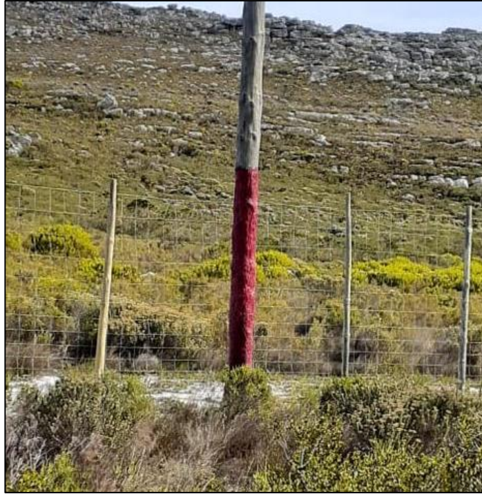
Figure 8. An electricity pole on Plateau Road treated with red grease, thus reducing the baboons' ability to reach the live wires.
