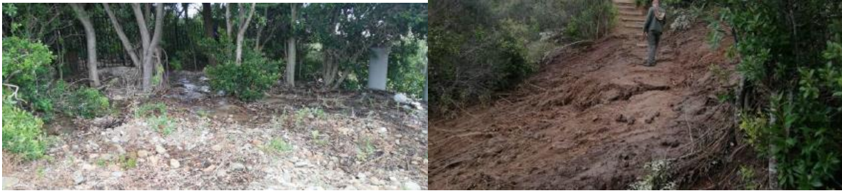
Figure 70: A pipe burst was reported by the Tygerberg NR staff on (19/12/19) around 10:00 and the pipe was only repaired after 16:00.
