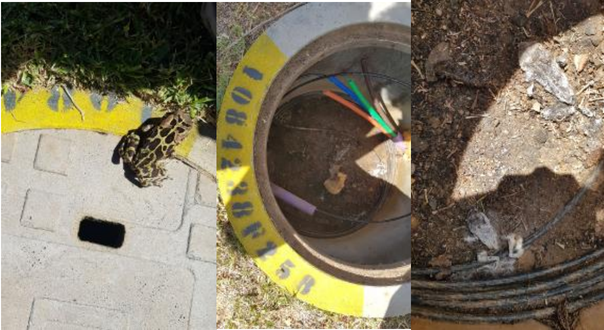
Figure 38: The fibre-optic manhole covers that create lethal pit-fall traps for the Endangered Western Leopard Toad in Constantia. One manhole contained 2 live adult toads and 4 dead individuals.
