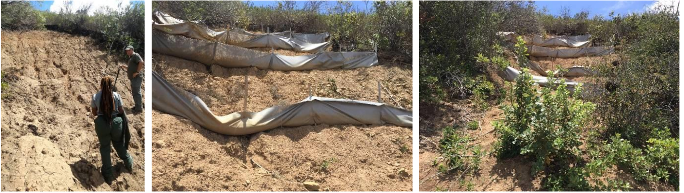
Figures 102-104: Impact of landslide erosion November 2019 (left). Silt curtains were installed in October 2020 (middle), aiding veld recovery, as seen in December 2020 (right).
