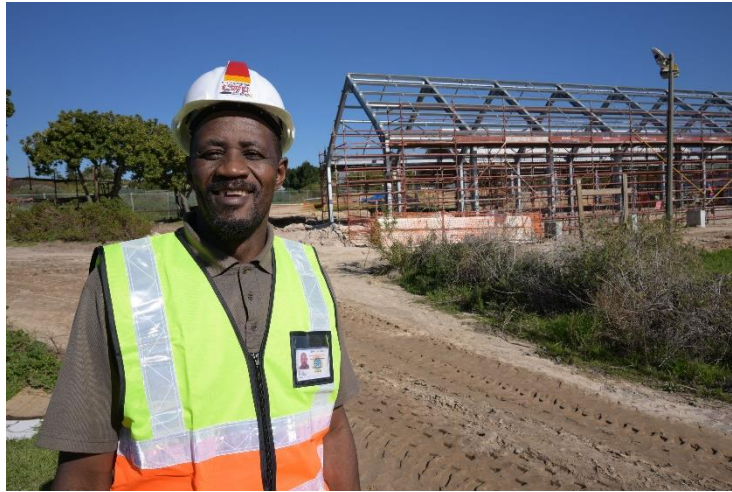
Figure 3: BMB staff member, Thobela Eric Bunu, with the Bracken Nature Reserve construction in the back ground.
