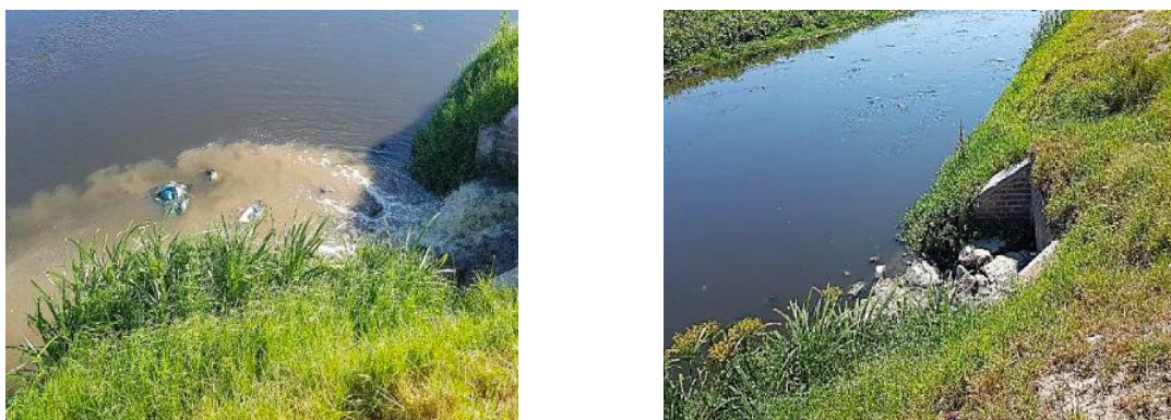
Figure 38: Bokmakierie pump station discharging raw sewage into the Blackwater river (left) and no discharge after the matter was attended to (right).
