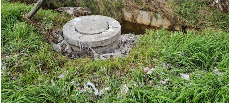
Figure 28: An example of manhole overflows directly entering the stormwater system and ultimately our natural watercourses.
