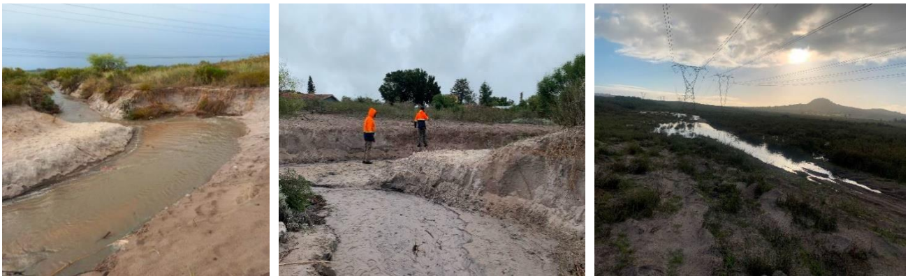
Figure 57: Soil erosion caused by the storm water manhole blockage at the Witzands Nature Reserve.
