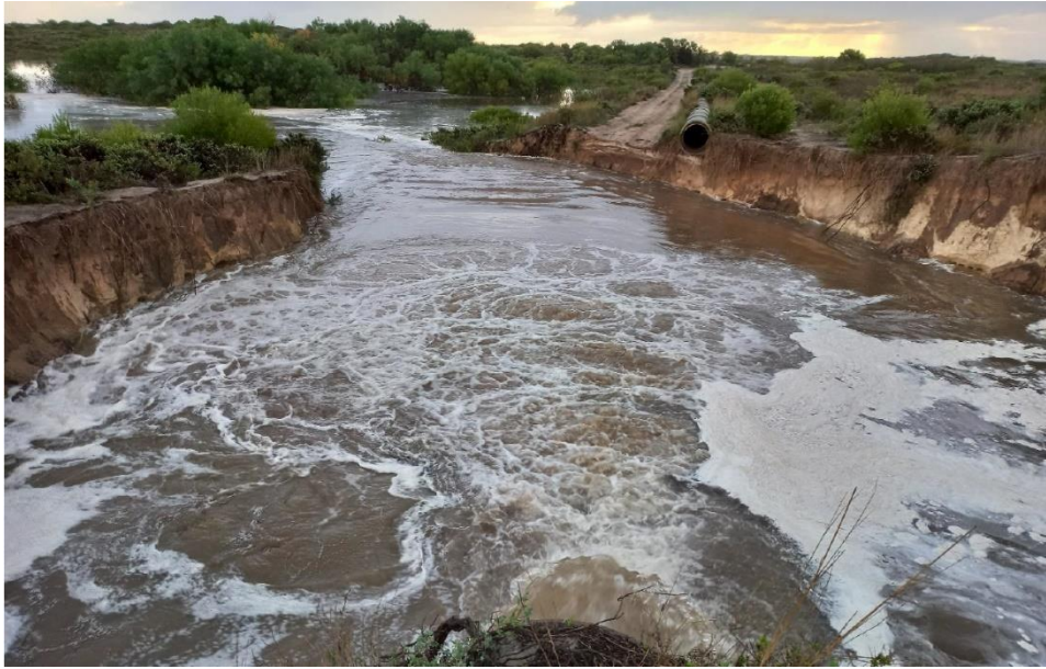
Figure 58: A large portion of the stormwater pipe leading to the urban storm water recharge pond (at Pond 7) collapsed on or about 14 June 2022.
