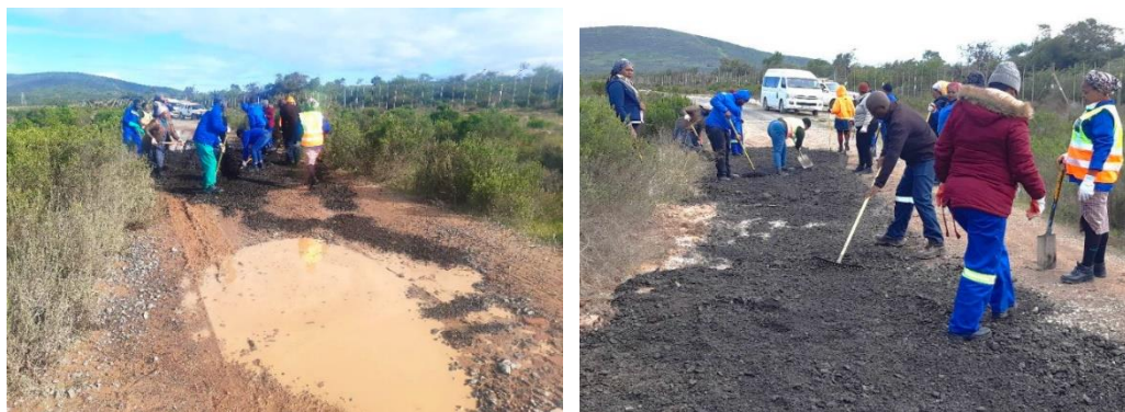
Figure 109: Portion of access road impacted by standing water (left) and milling material used to fill and level the road (right).
