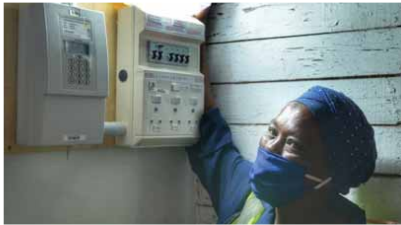
A turn-on: In May, the City switched on electricity to 48 households in the Smallville informal settlement in Schaapkraal, Philippi. Ms Josephine Saunders (pictured) is one of the beneficiaries of the R800 000 electrification project.
