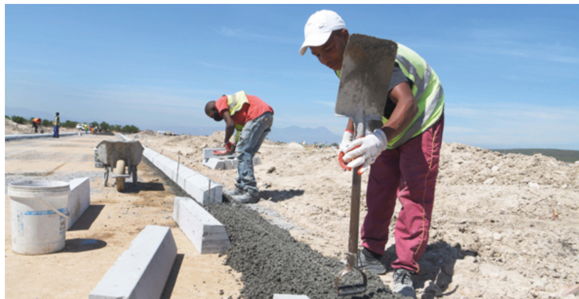
Crafting kerbs in Macassar housing project: Construction of civil engineering services is under way at the City's mega Macassar housing project. The development will eventually house 2 469 beneficiaries. The civil engineering contract is being completed in three phases. Phase 1 comprised the civil works for 605 erven and was completed in April 2021. Civil works for phases 2 and 3 will be completed in October 2022 and June 2023 respectively. Beneficiaries will be selected based on the City's Housing Allocation Policy and Housing Needs Register to ensure fair and transparent allocation of housing opportunities and prevent queue jumping. Help the City protect its housing projects by reporting illegal activity (such as unlawful occupation) at 021 480 7700.
