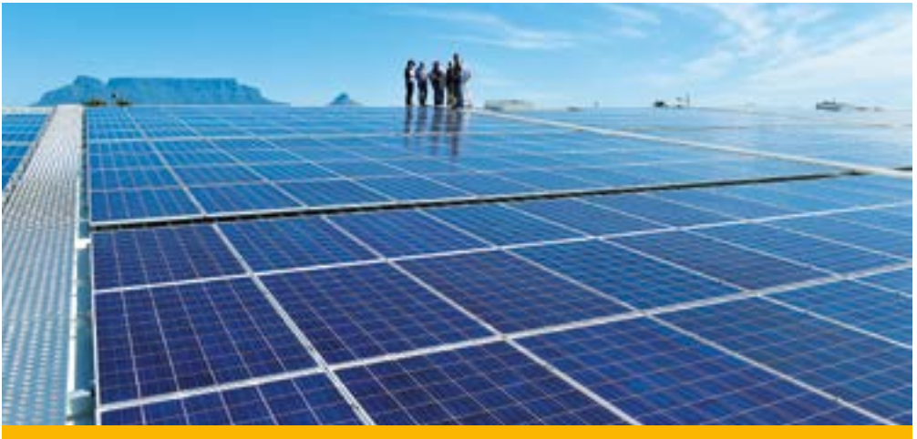
Grid-tied PV system at Bayside Mall.
