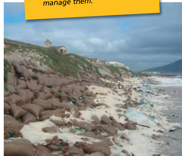
Sandbags fail to stabilise the dunes at Dolphin Beach.
