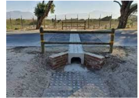
Toad tunnels are being trialed adjacent to False Bay Nature Reserve to assist toads to reach their breeding sites safely.
